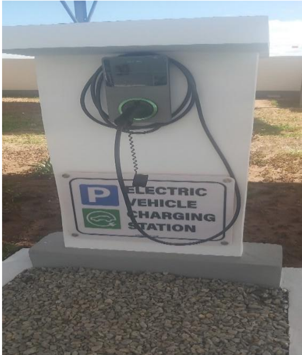
Figure 4: Example of an accessible residential charging station
