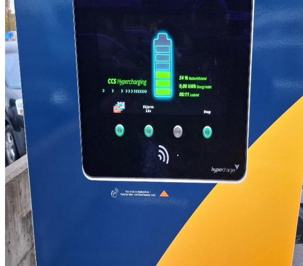
Figure 3: 150KW CCS Charger
